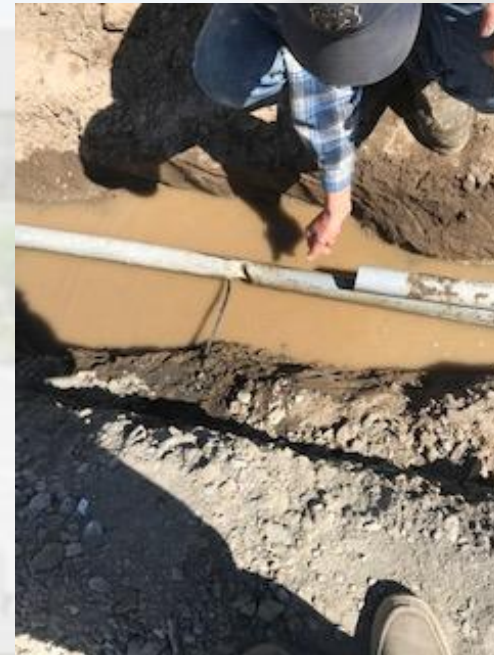
Picture shows section of pipe that had to be replaced (top pipe) and Fiber optic conduit that was cannibalized by utility company
